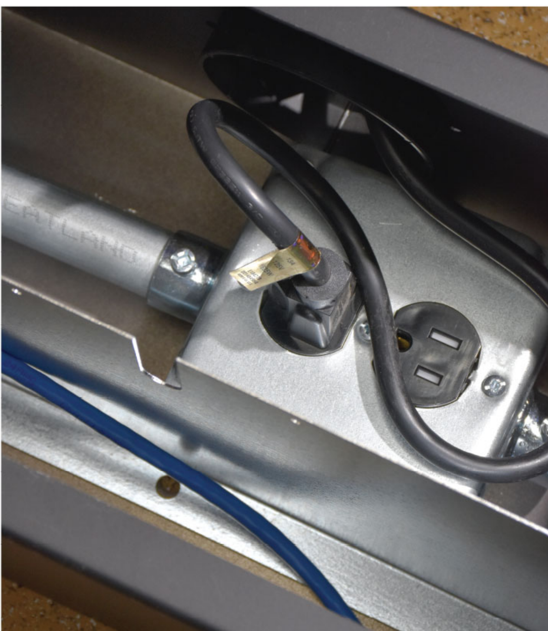
Isolates Different Voltage Cords/Conduit/Cables >>>
